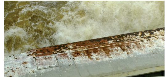
Vinyl coating in poor condition due to abrasive action of debris-filled swirling water
